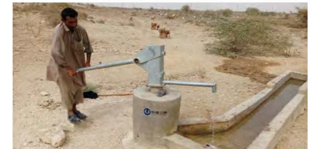
A water supply facility improved by CSAIL
